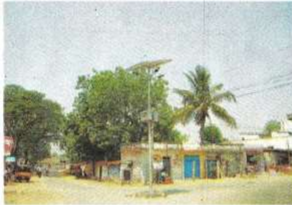
A file photo of the solar LED street lights in Chigurumamidi mandal in Karimnagar. RM DAYASHANKAR
