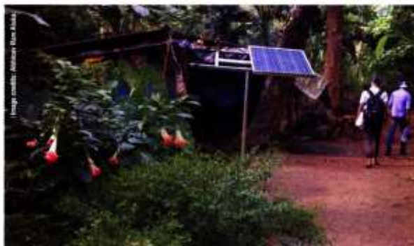
A home in Kundhal, a village near the Nellore town, running on Solar-DC Inverterless
