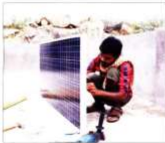
Local entrepreneur installing Solar-DC Inverterless in a home in Jang Thakur hamlet in Nagpada, Telangana
